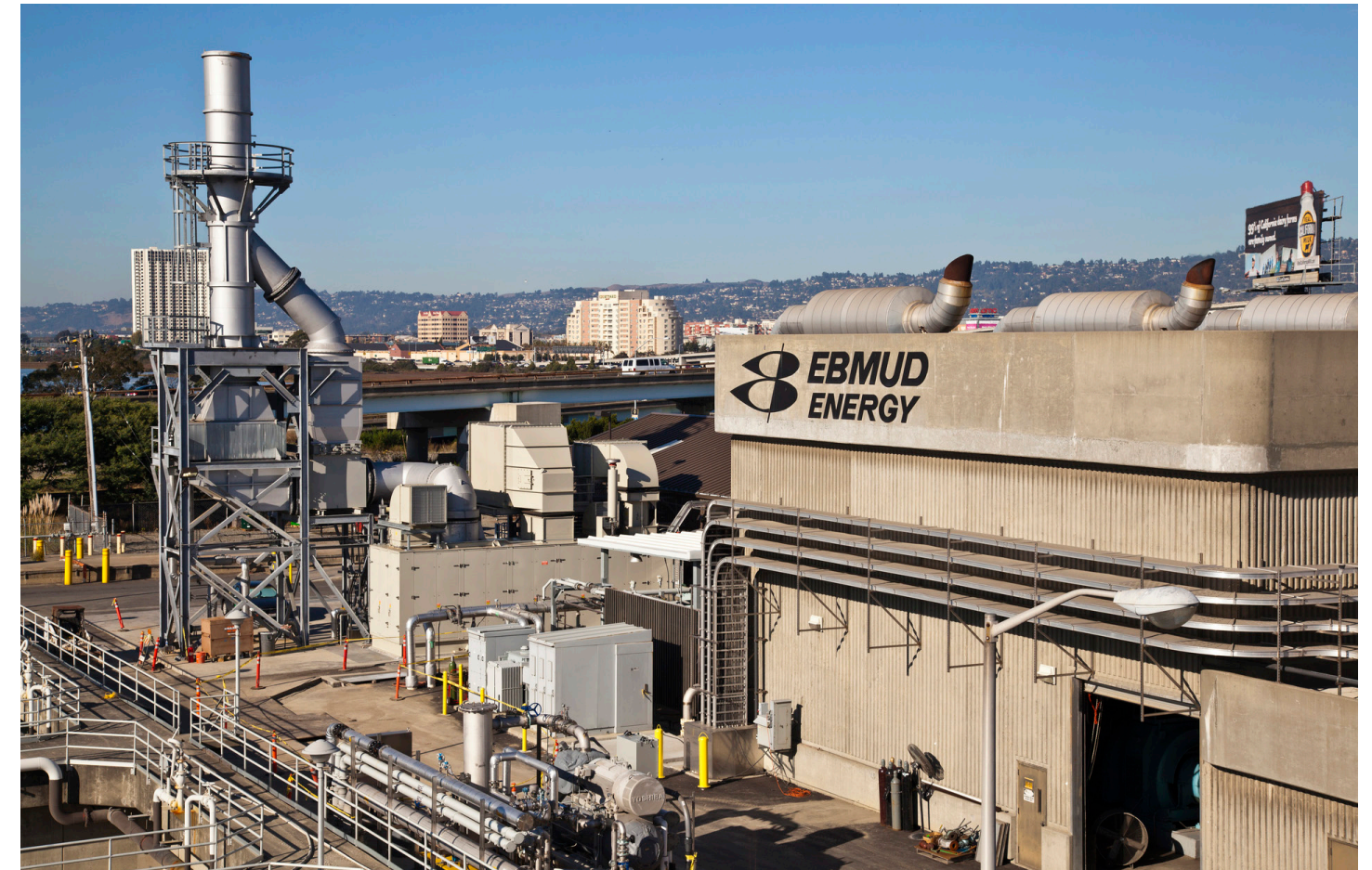
Overaa, "EBMUD energy plant," 2020.
