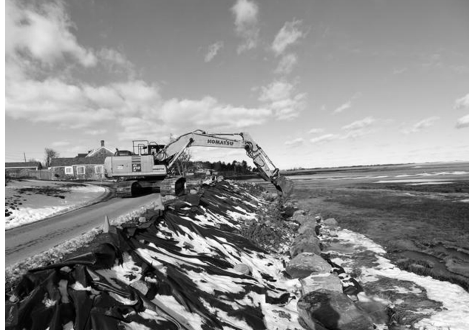
Paul Bilodeau, Work on the Seawall at Conomo Point in Essex has begun , 2022, Photograph, Essex, Massachusetts
