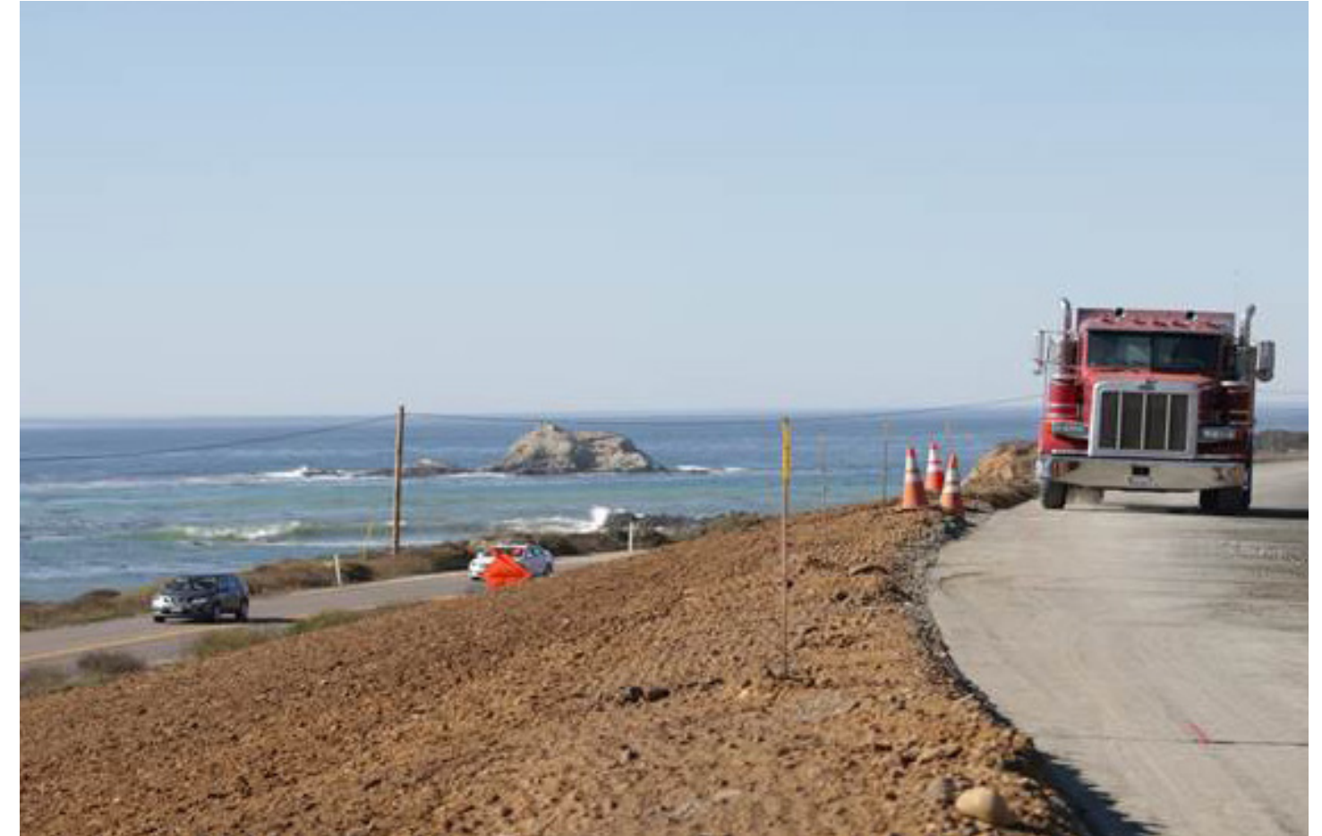
Jim Shivers, "Existing lanes of Hwy 1 with grading for new lanes", Big Sur Blog , 2017
